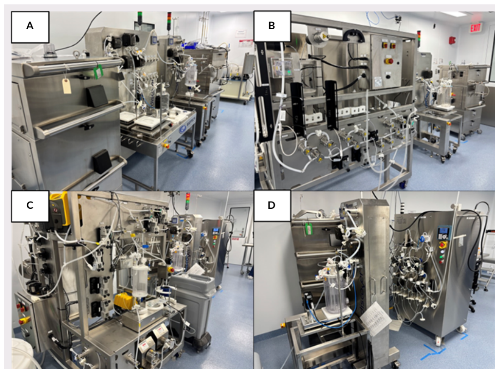
(A) IVTR and PIVT skids, shown installed with the associated PAT Box skids post-commissioning, used for real-time monitoring and control of transcription reactions. (B) Chromatography skid, employed for purification of mRNA intermediates. (C) Drug substance TFF skid, used for tangential flow filtration and buffer exchange of the purified mRNA. (D) LNP formulation skid, for encapsulation of mRNA into lipid nanoparticles suitable for drug substance production. DSTFF: drug substance TFF; IVTR: in vitro transcription reactor; LNP: lipid nanoparticle; PIVT: post-IVT; PAT: process analytical technology.
